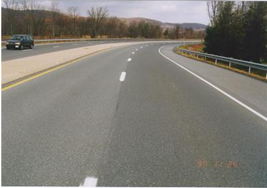
Photo 7. Lehigh County, Saucon Valley Road Westbound travel and passing lanes at Sta 27+50 looking west, control section without shingles on 11/24/97.
