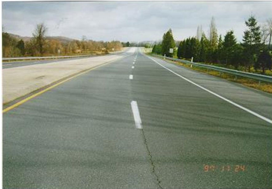
Photo 8. Lehigh County, Saucon Valley Road Westbound travel and passing lanes at Sta 34+00 looking east, control section without shingles on 11/24/97.
