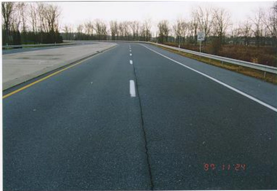
Photo 6. Lehigh County, Saucon Valley Road Westbound travel and passing lanes at Sta 36+90 looking west, with shingles in both the wearing and binder courses on 11/24/97.
