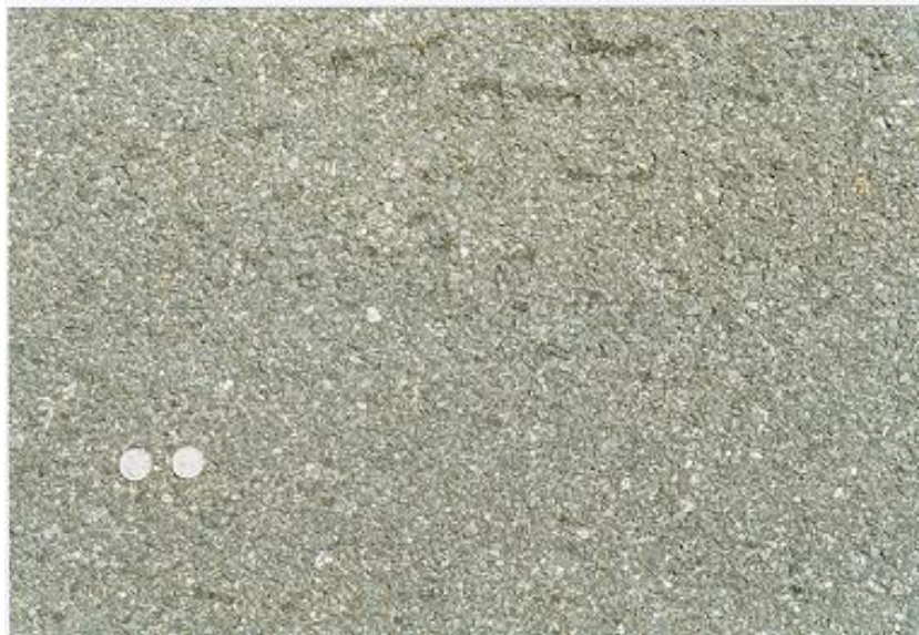
Photo 4. Lehigh County, Saucon Valley Road Close-up view of the bituminous concrete with fiberglass asphalt shingles in ID-2 wearing course at Sta 36+90 in 1995.
