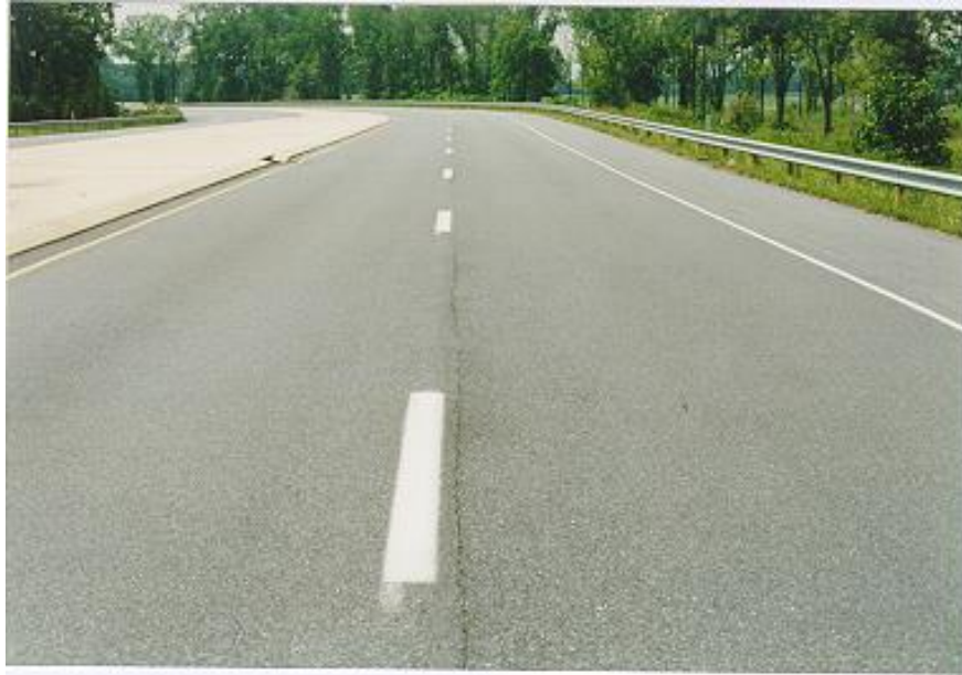
Photo 5. Lehigh County, Saucon Valley Road Westbound travel and passing lanes at Sta 36+90 looking west, with shingles in both the wearing and binder courses on 8/17/95.
